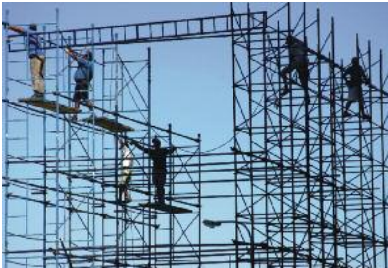
Dangerous construction site. Author: Peter Rimmer
